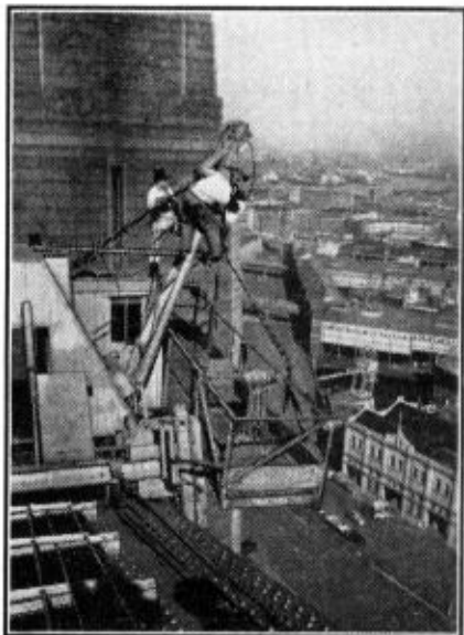
Sidney Black and Ernest Tomrup are quite at ease overhauling the hoisting wires of a painting stage 250 ft. above sea level.
